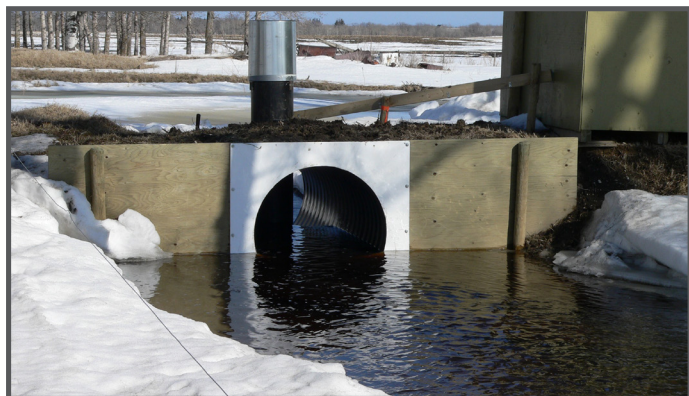
Circular flume at monitoring station Ms6
