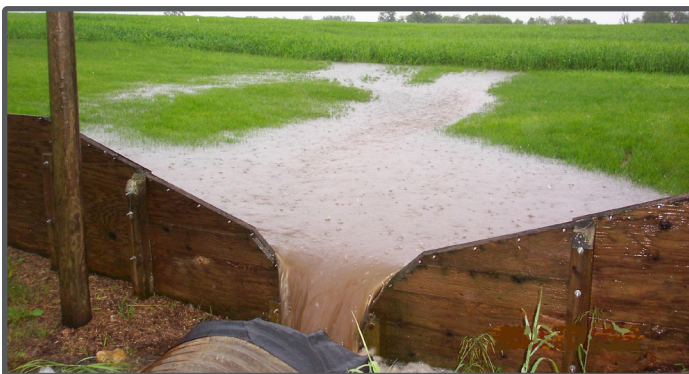
V-notch weir at monitoring station Ms11
